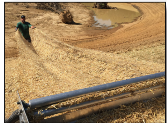
UnReel Installer shown in 8' length (top), and facilitating installation down a steep slope (bottom).
